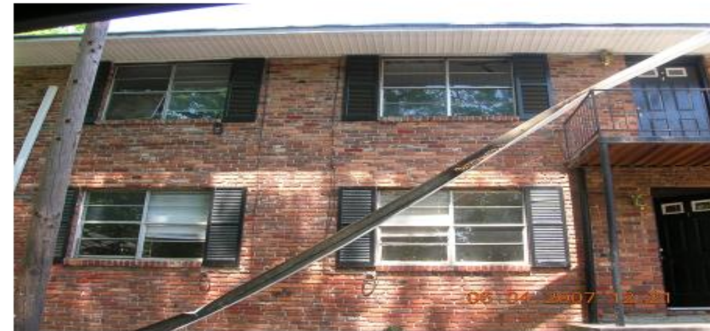
Gutters Hanging Off of Building
