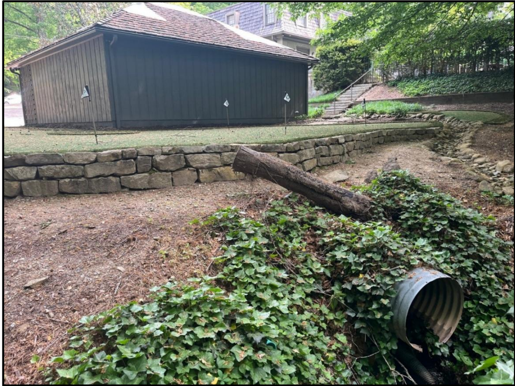
View of the rear of the existing two-car garage and the corrugated metal pipe upon which it sits
