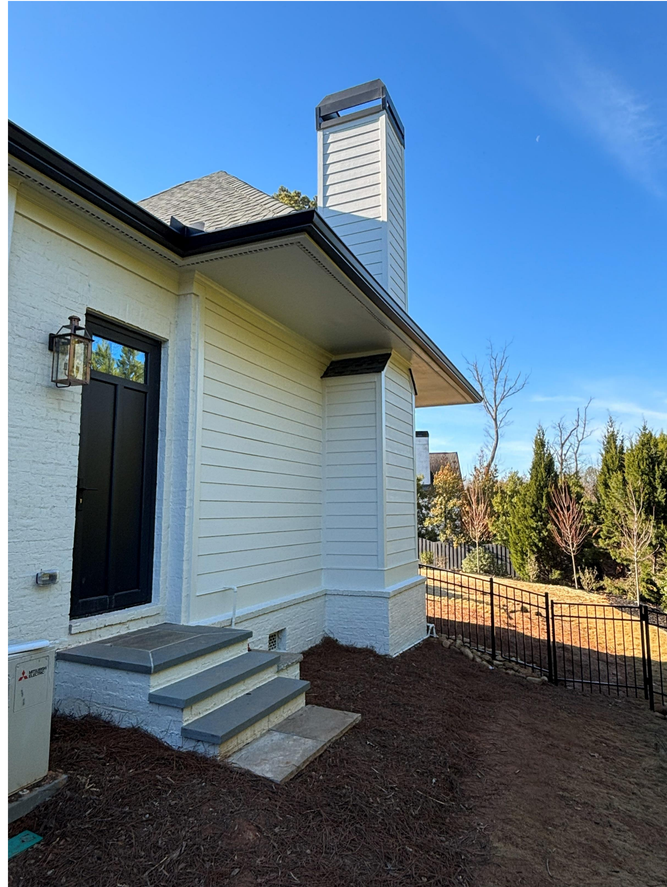
View of building eave encroachment facing Southwest
