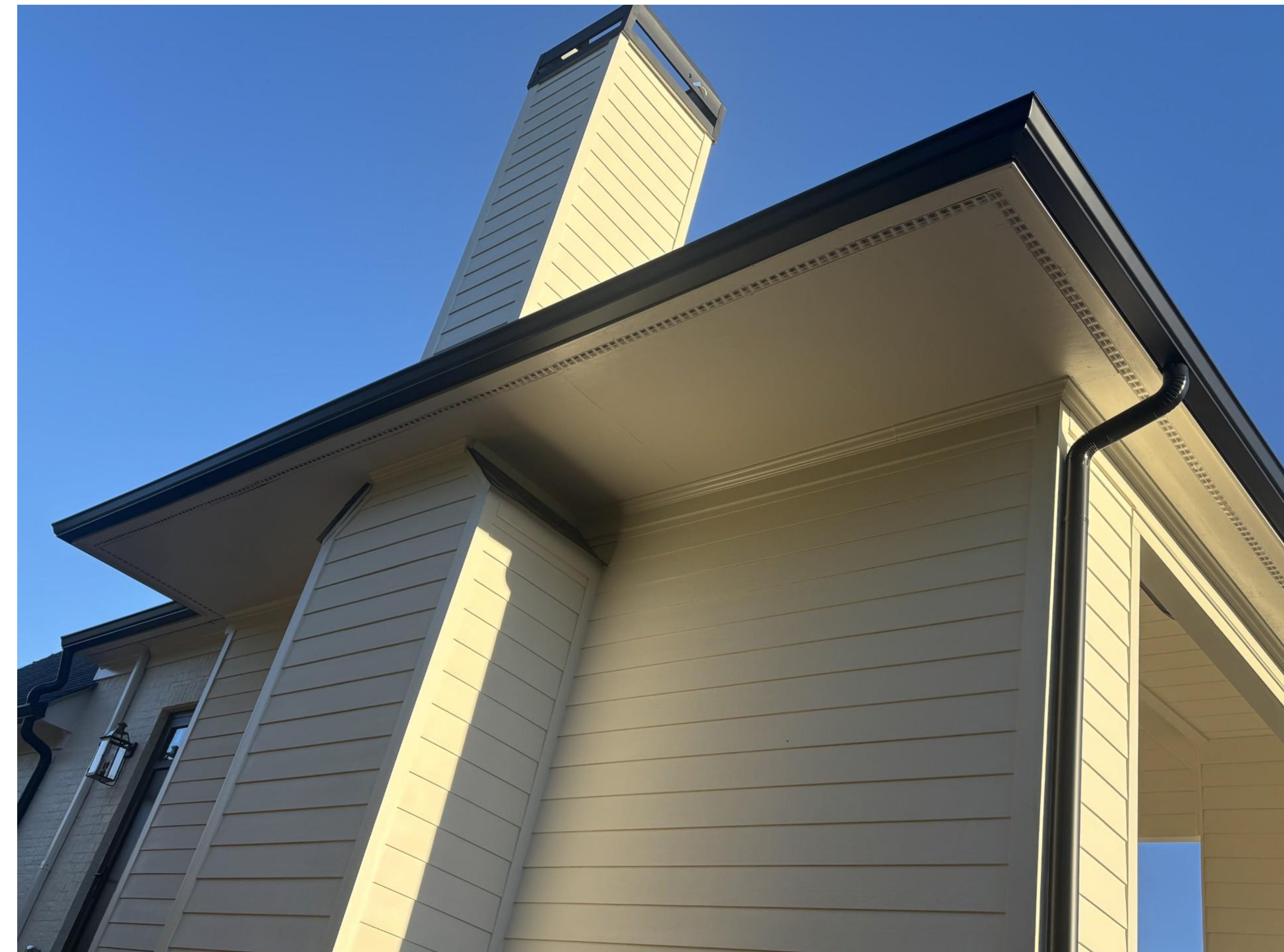
View of building eave encroachment facing South
