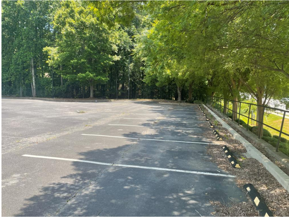
View of parking lot in front of bank – Roswell Rd is to your right
