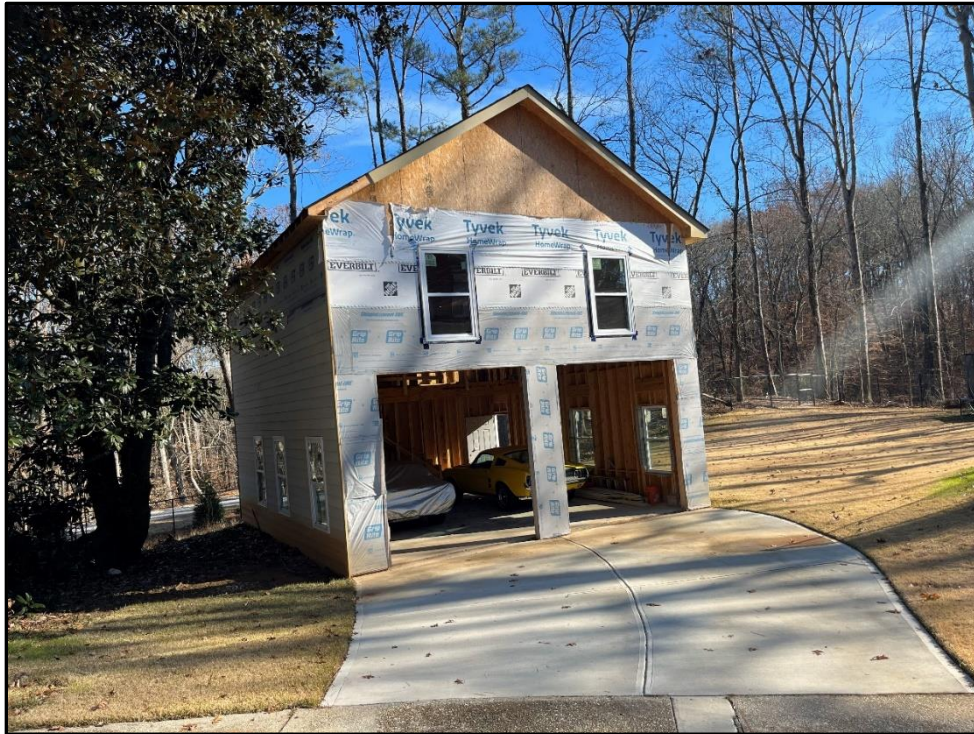
View of unpermitted garage on Skyridge Trail
