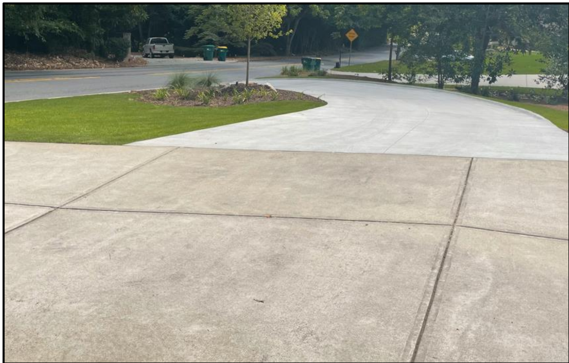
View of noncompliant driveway facing east
