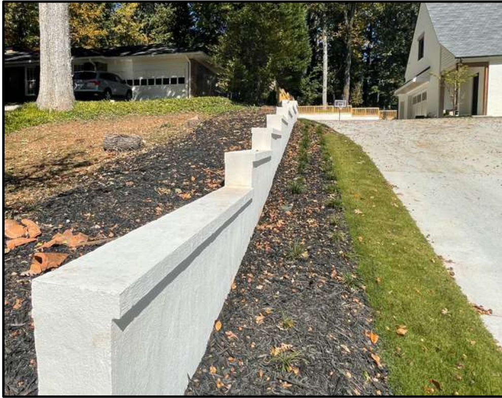
View of noncompliant retaining wall standing on Forrest Lake Drive looking north
