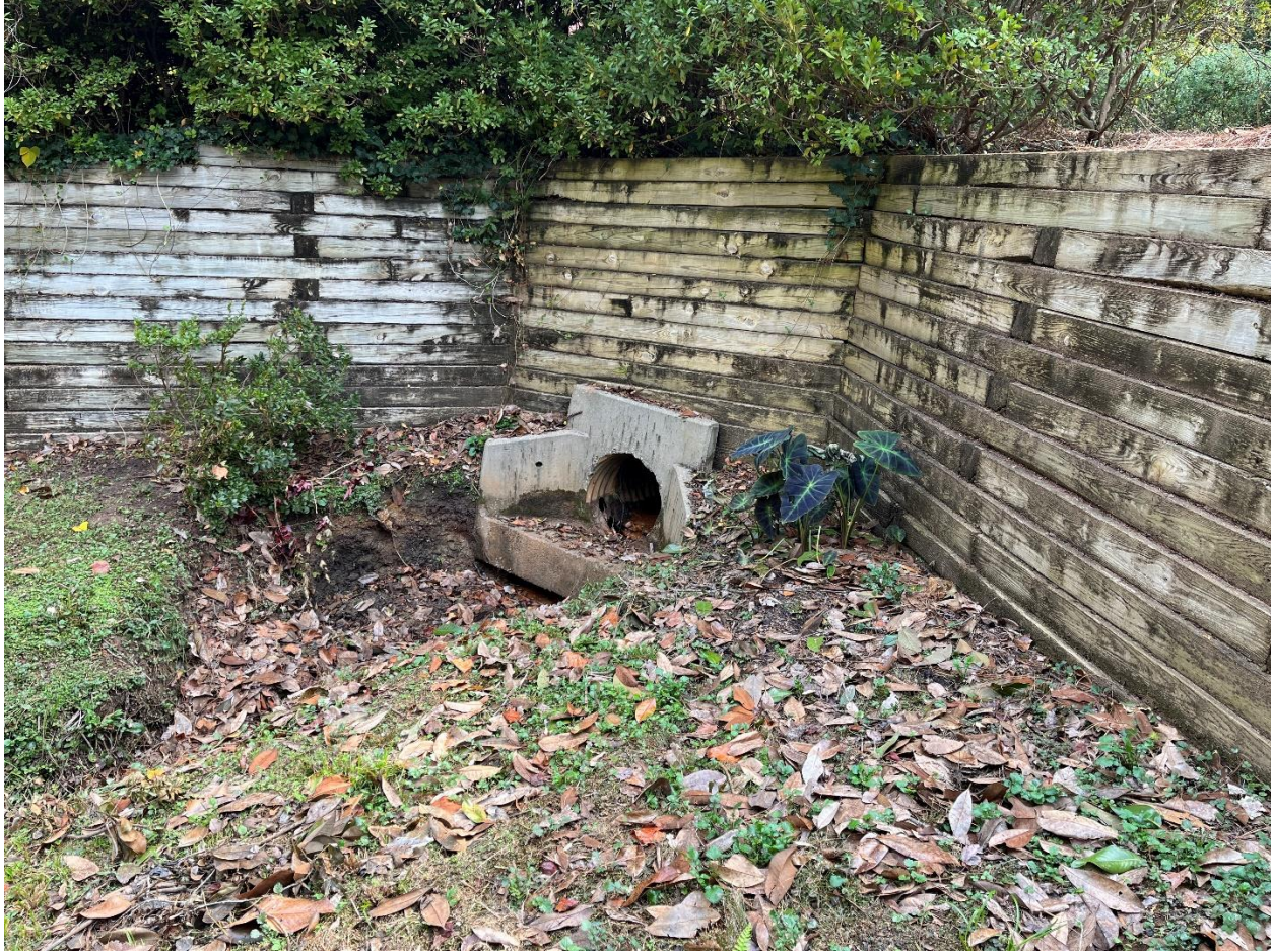
View of Downhill side of pipe & wall, repairs will be made to secure outfall area
