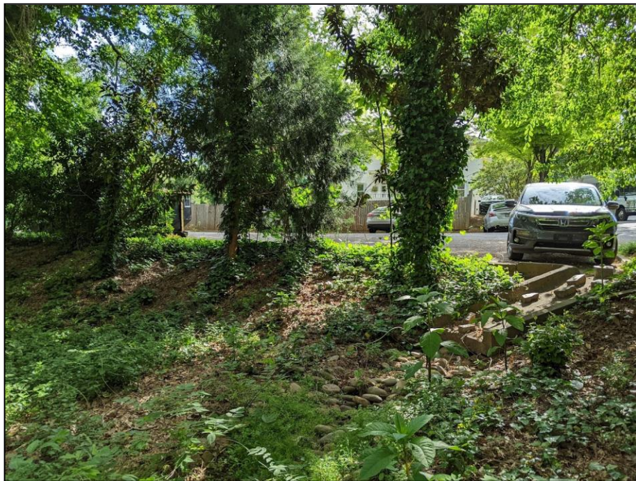
View facing east, from within vegetative dry detention facility; concrete flume to the right where stormwater enters
