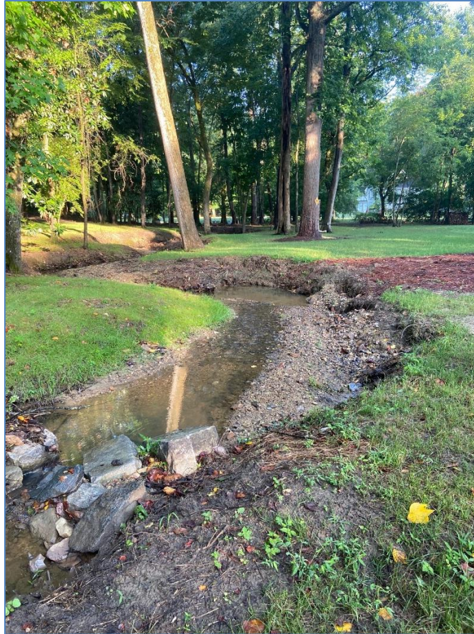
Portion of the stream which is eroding
