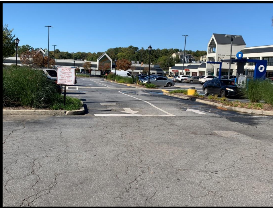
Photograph 14 – Parkside Shops East Parking Lot Incorrect Striping Colors
